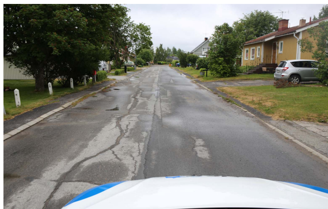
Fig. 2. Residential street in need of reconstruction (black category segment), located in Skellefteå municipality. (Image courtesy of Skellefteå Municipality.)
